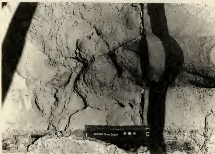
Fig. 26. Cracking and displacement of tuff at cornice level at east wall of apse (Photo: Anne Brackin).
